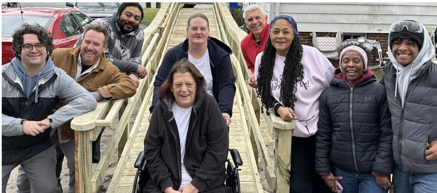
Salisbury Christian School students and members of the Wicomico Rotary Club work together to build a wheelchair ramp for Mary S. of Salisbury on April 12, 2025.
